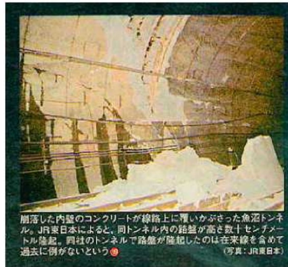
Figure 15 Big damage for Uonuma Tunnel
