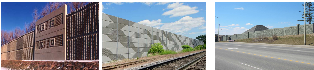
Figure 3 – Durisol noise barrier panels in service
