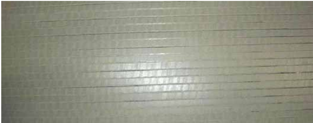
Figure 3 – Dry Saw Cut Edge Appearance
