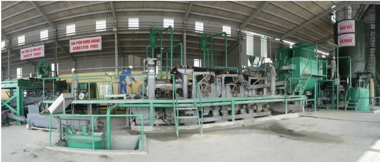
Figure 8 - Main equipment of non-asbestos cement production line at TTC
