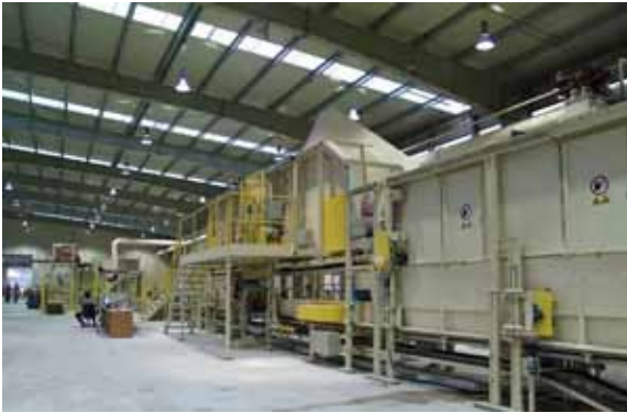
Figure 7 - Fully-automated Phase IV WWCB Plant
