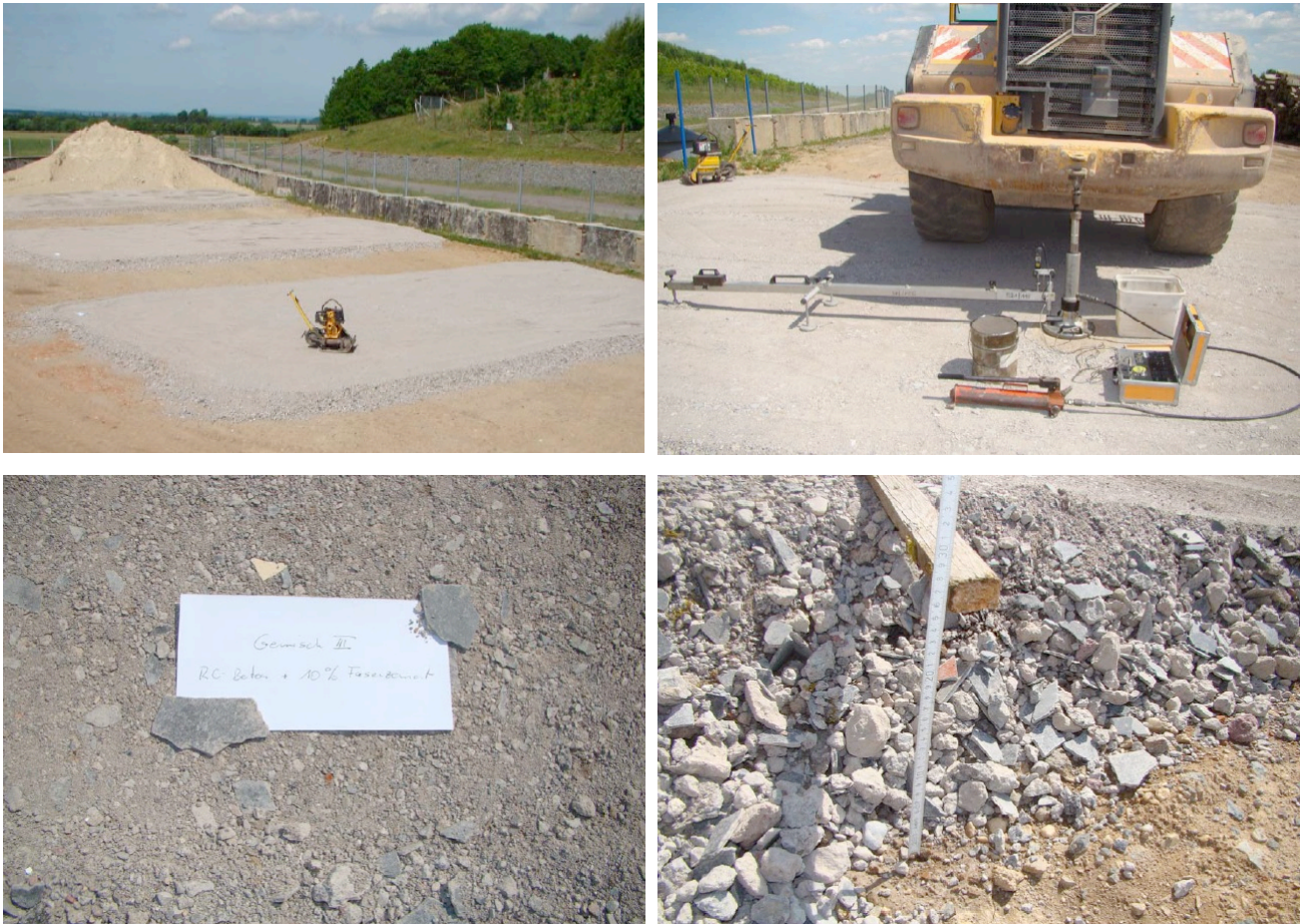
Figure 5 – Real scale road basement test with mixture composed of concrete rubble and 10 weight% crushed FC
