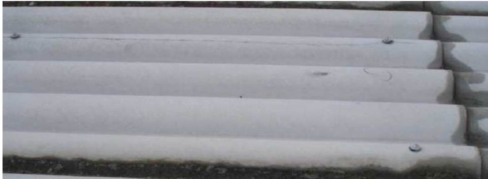
Figure 6 - Typical wet dry crack happen to 90% at the fixing point
