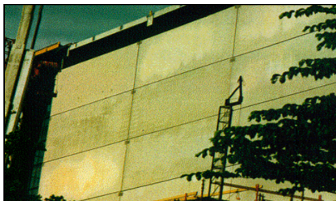
Figure 11 - Extreme staining at some elements in Norway (Häring 2003)
