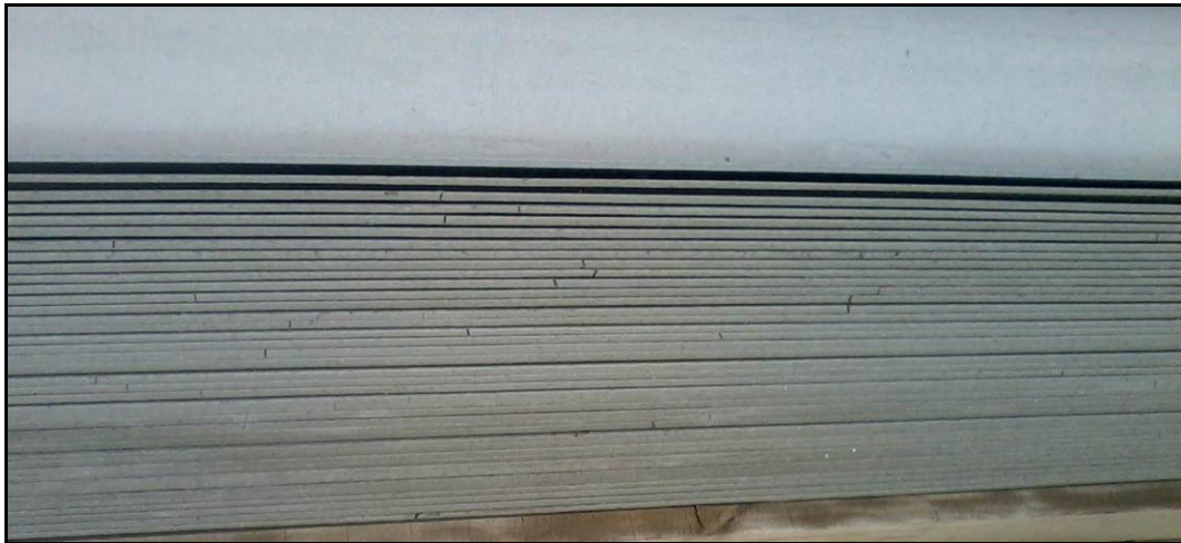
Figure 7: Kaolin modified corrugated sheets cured outside, without plastic wrapping, showed wide edge cracks after 30 days curing.
