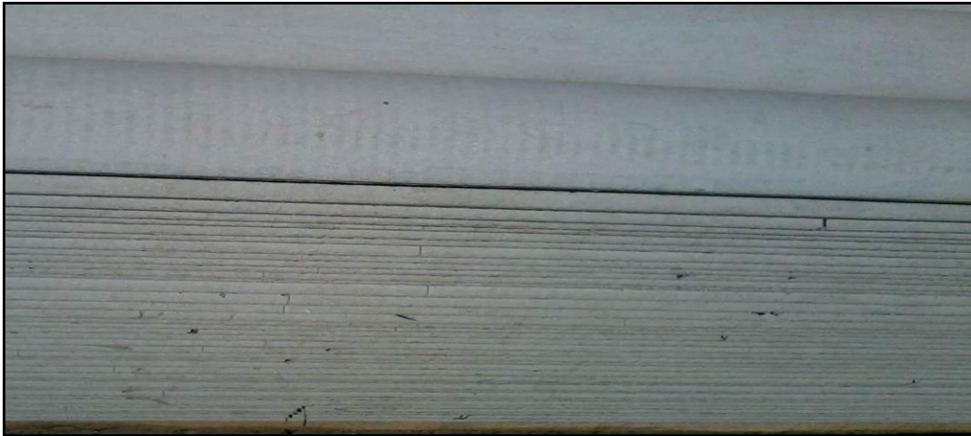
Figure 6: Corrugated sheets stored internally, with plastic wrapping, then cured outside without wrapping. Edge cracks appeared after 30 days curing period.
