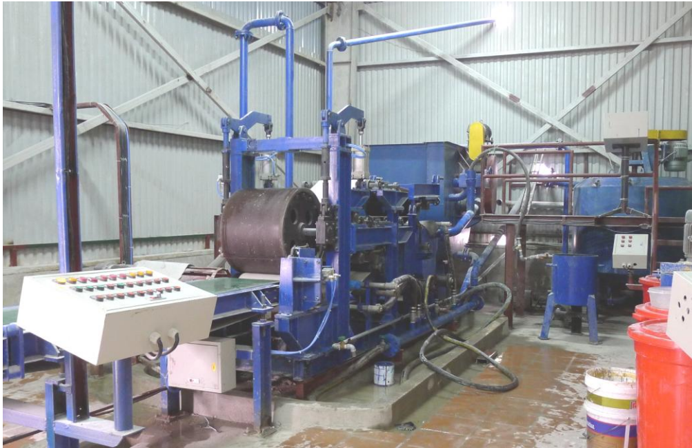
Figure 5. Panorama of mini Hatschek line installed at site.
