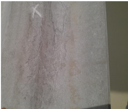
Figure 6- Cracks on the PCA-C sheet
