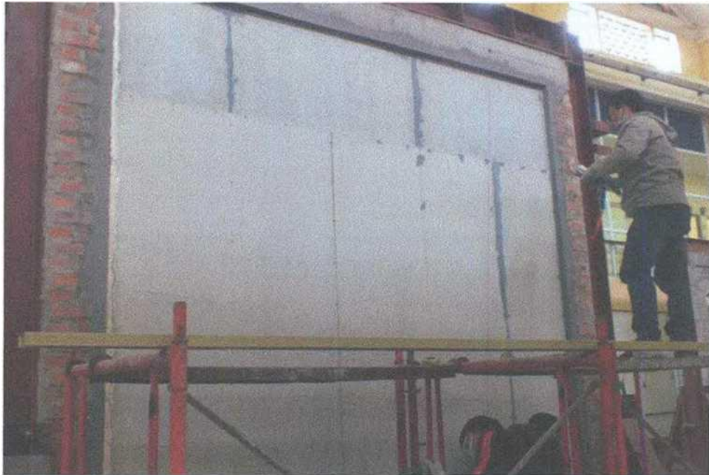
Figure 9: Installation of DURaflex boards (outer layer-10mm) on the exposed face of test specimen
