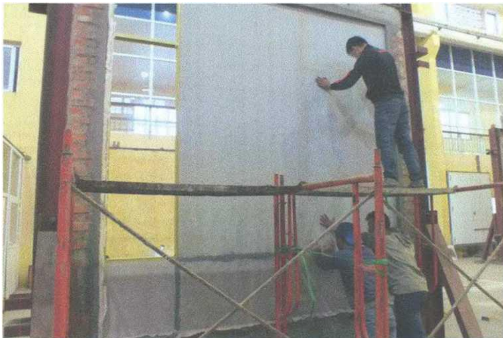
Figure 8: Installation of DURA flex boards (inner layer-6mm) on the exposed face of test
